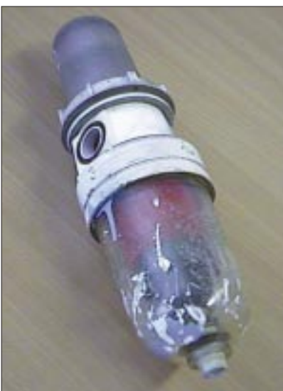
Figure 16. Filter removed from a breathable air set in an automotive paint shop.
