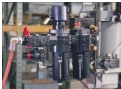
Figure 14. Use of a lockable tamper evident cover on a filter/regulator.
